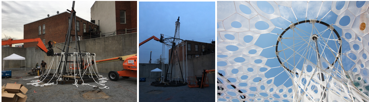
Figure 8: Erection sequence: ring laced (left); ring laced with top connections (center); Fully installed [photo courtesy: Pablo Enriquez] (right)
